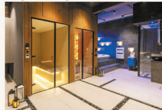
Spa Wet Area Equipments
